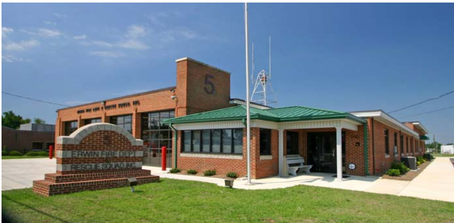
“The Erwin Fire Station renovation required construction staging in order for vehicle bays to remain operational.”
