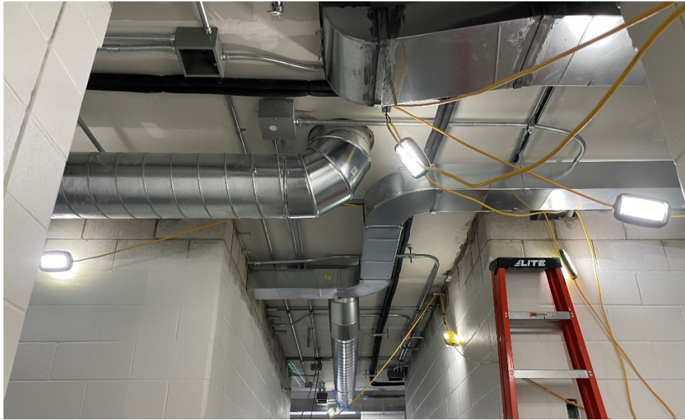
Corridor Ductwork Installed
