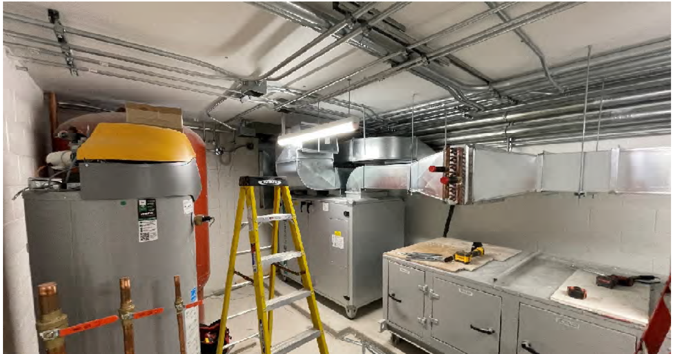
Mechanical Room Equipment Installed
